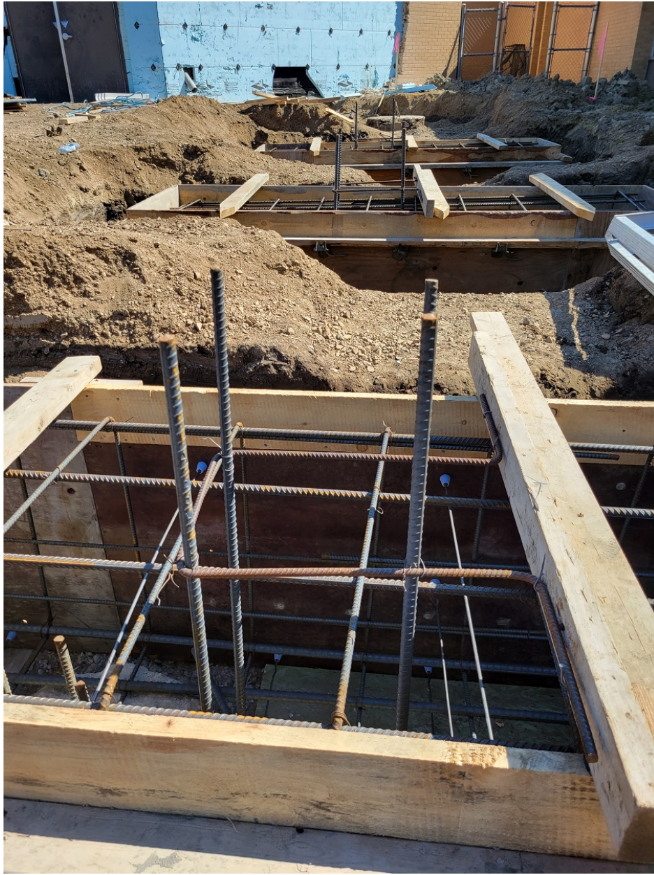
Photo #03 – Pile caps along Grid Line 2 looking from Grid Line E east
