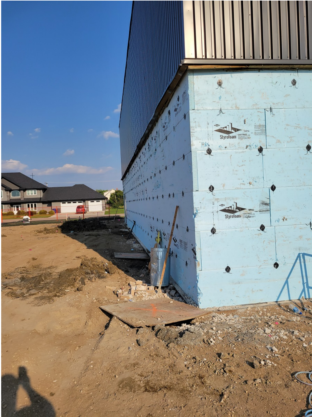
Photo #06 – North east corner of existing gym brick removed with piles covered.
