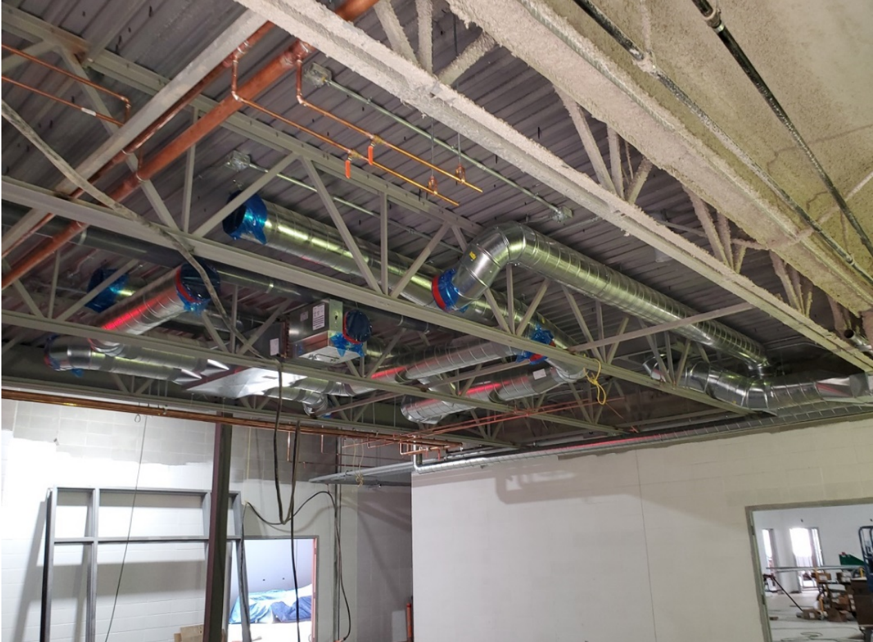
Photo #6 – Mechanical on Main Floor
