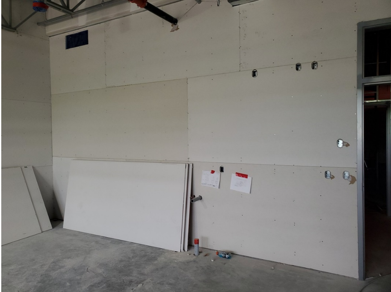
Photo #8 – Second Floor Classroom Drywall
